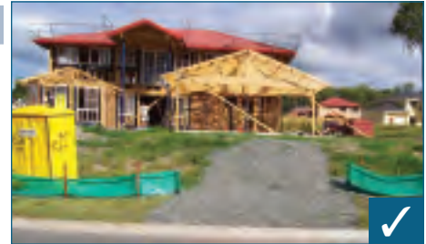
Stabilised gravel entry/exit point (rumble pad)
