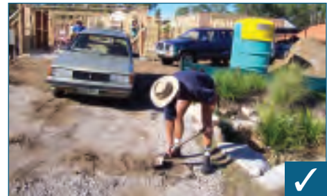
Excessive sediment deposits must be removed from entry/exit point (rumble pad) and additional crushed rock applied
