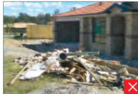
Poor litter and building waste storage
