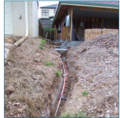
Service trenches should always be backfilled, capped with topsoil and compacted
